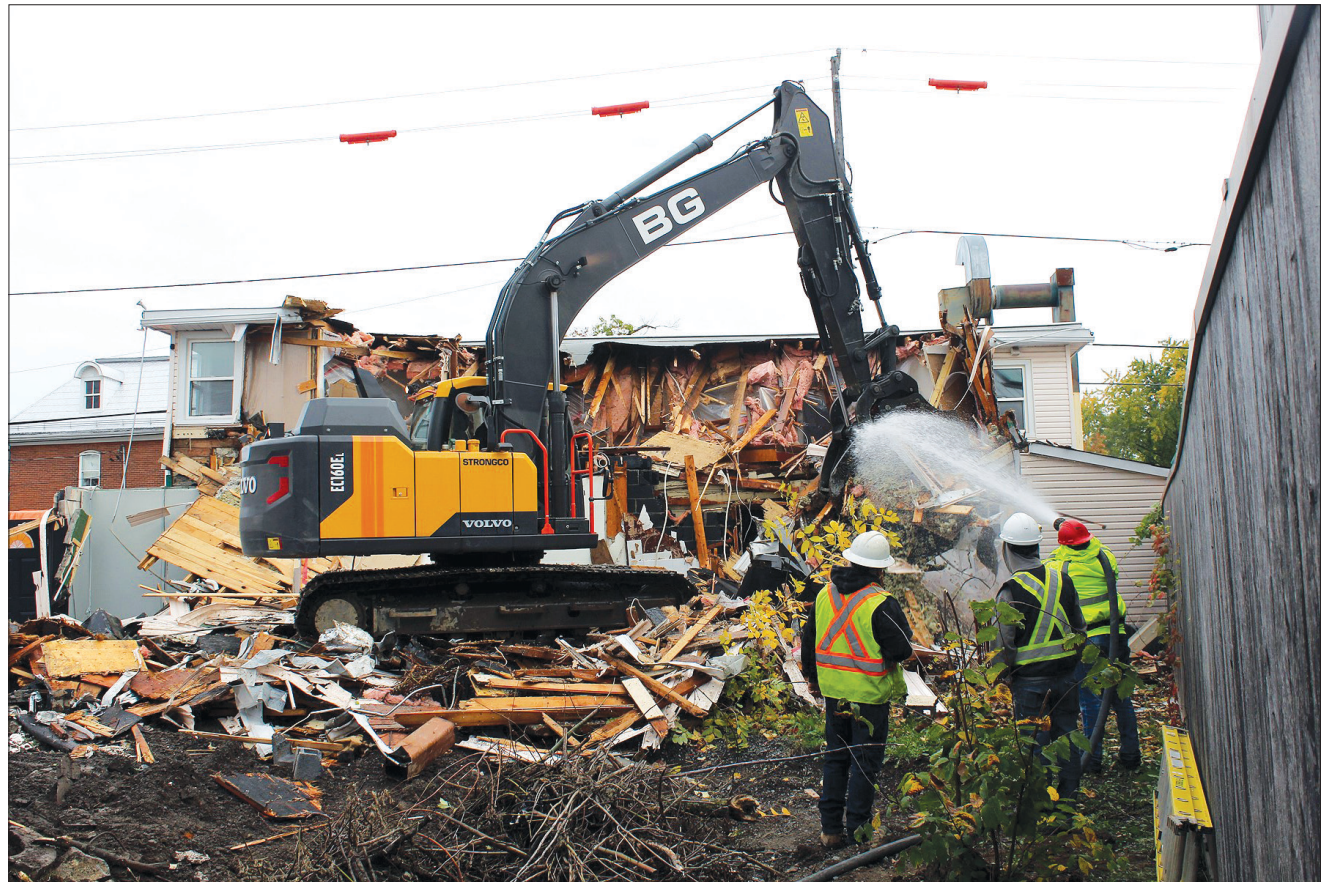
Workers tear down the old Manotick Tea Room building last week. The condemned building had stood since 1865. It will be the site of a new two-storey office building for Royal LePage Team Realty. GREG NEWTON PHOTO
