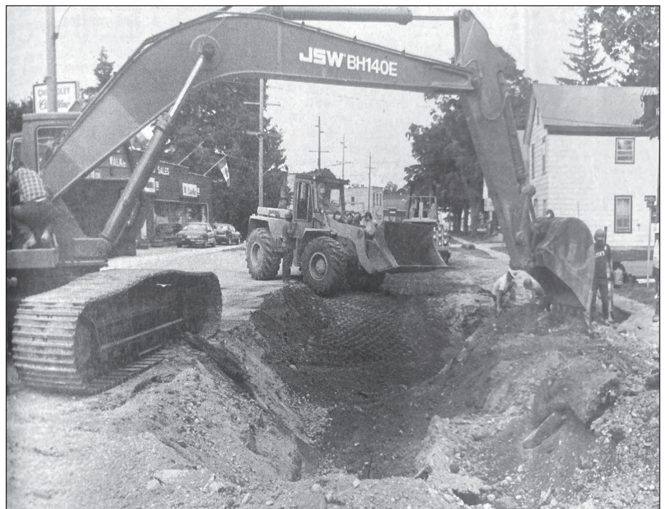
From the July 11, 1990 issue of the Herald-Times Construction on Durham Street, Walkerton, is expected to last until mid-September as crews install a new watermain.
